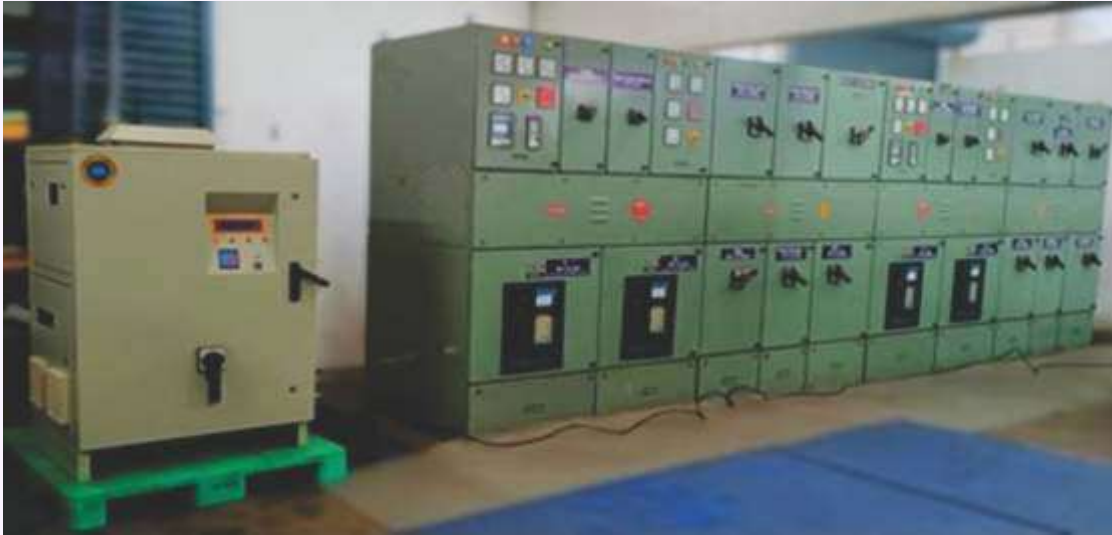
50 kVA STATCOM installed in industrial premises
