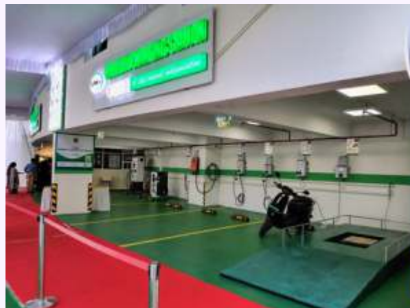
Model Charging Station (MCS) at C-DAC Thiruvananthapuram
