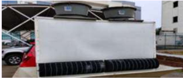
30 kW Panel Water Cooler installed at IISER, Pune
